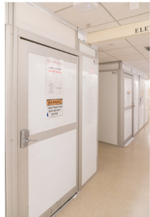
Figure 1. Image of a hallway in a hospital where construction is taking place. Warning signs on the doors act as barriers to contain dust and debris.
